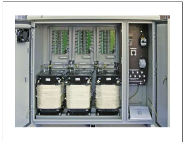
Internal view of an Outdoor Isolating AVR
